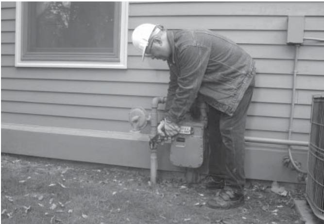
Figure 1.7 — Manual Shutoff Valve
